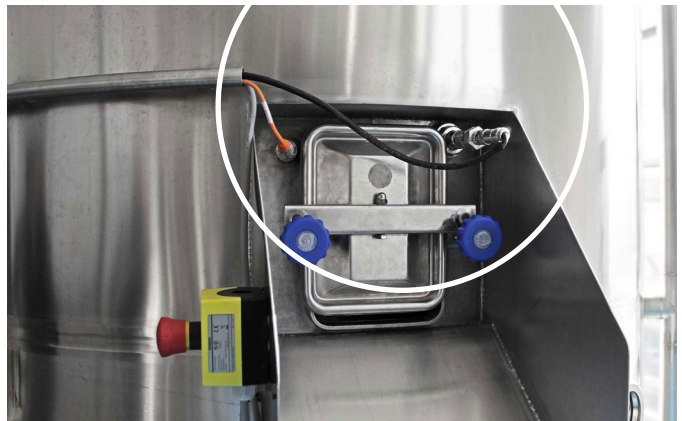
A TS Temperature Sensor (flush) and the upper pressure probe of the D3 Differential Pressure Sensor monitor the lauter tun.
