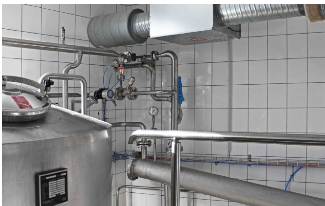
The vapor recompressor: the heart of energy recovery with TS Temperature Sensor and HH Pressure Sensor in the wort boiler
