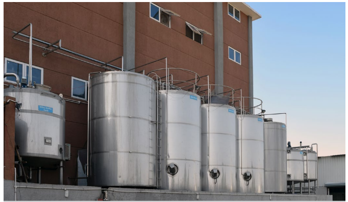
The CIP plant with sensor technology for conductivity measurement (ILM-4) and point level (NCS-11), ensuring a maximum recovery of the return of rinse water, acid, and lye. The multiple use of resources helps saving water, energy, and detergent cost. TS temperature sensors and FMQ flow sensors complete the sensor range.
