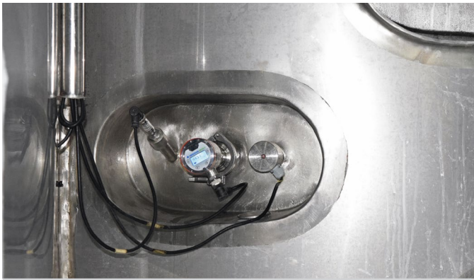
Storage tank monitoring with L3 pressure sensor, NCS-11 level switch and TS temperature sensor
