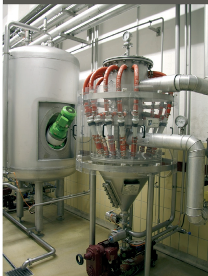
Figure 1: Left: Storage tank for the tartar seed crystals, front: Venturi centrifuge
